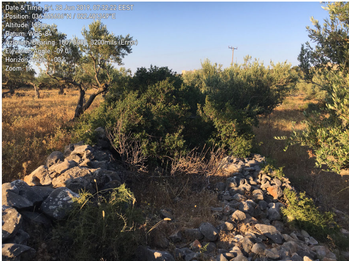
Fig. 9. Geotagged photo from Leg 10 (Kouloumi to Mezapos). This section of the walled footpath was impassable due to vegetation growth.
